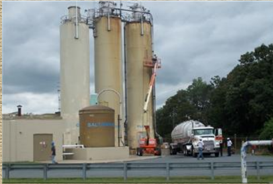
Distance shot of silo 3 being water blasted with operator using an 85 foot articulating boom
